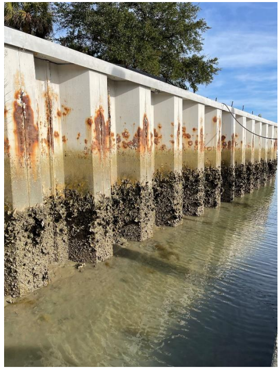
018-view of bulkhead at low tide, note marine growth and corrosion Station 22+00
