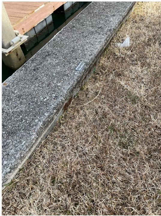
007-backfill subsidence Station 43+00
