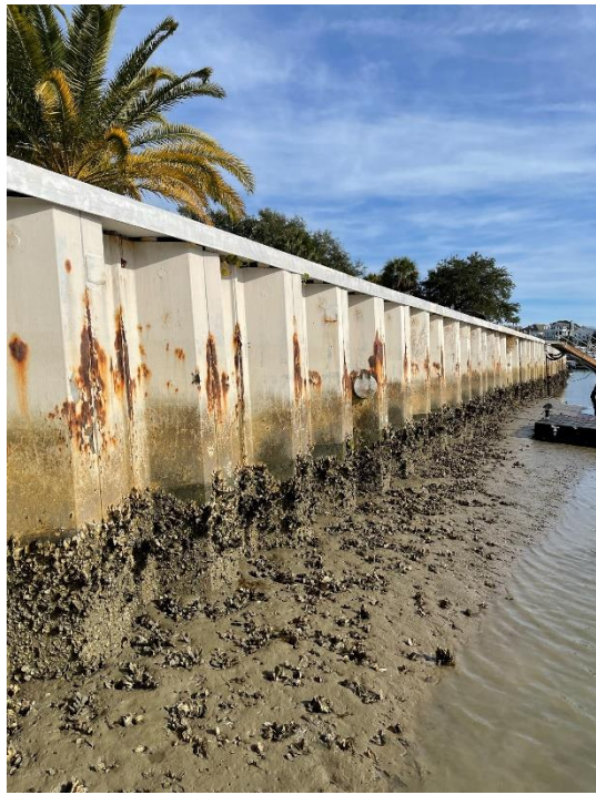
017-view of bulkhead at low tide, note marine growth and corrosion Station 22+00
