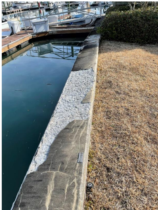
003-deterioration concrete cap, aggregate exposed Station 59+00
