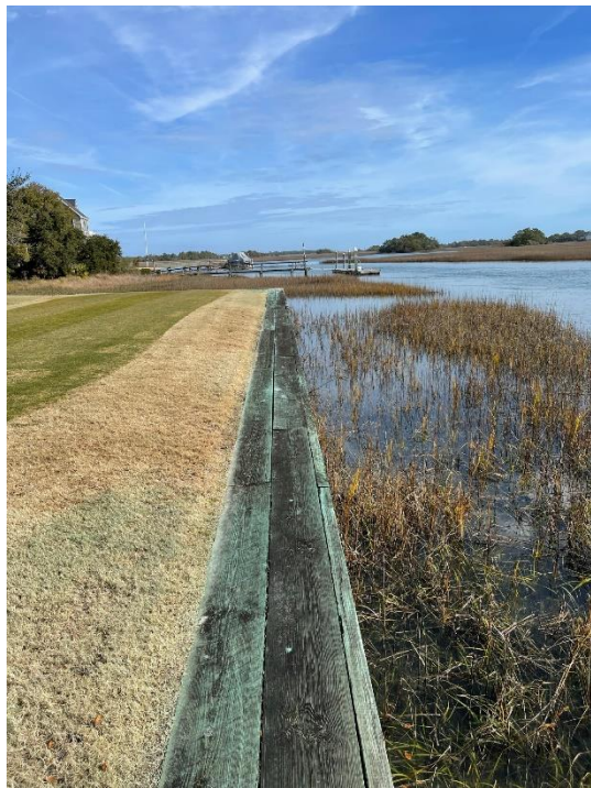
015-1 WWI, the shoreline is covered with well-established vegetation. No evidence of erosion along shoreline
