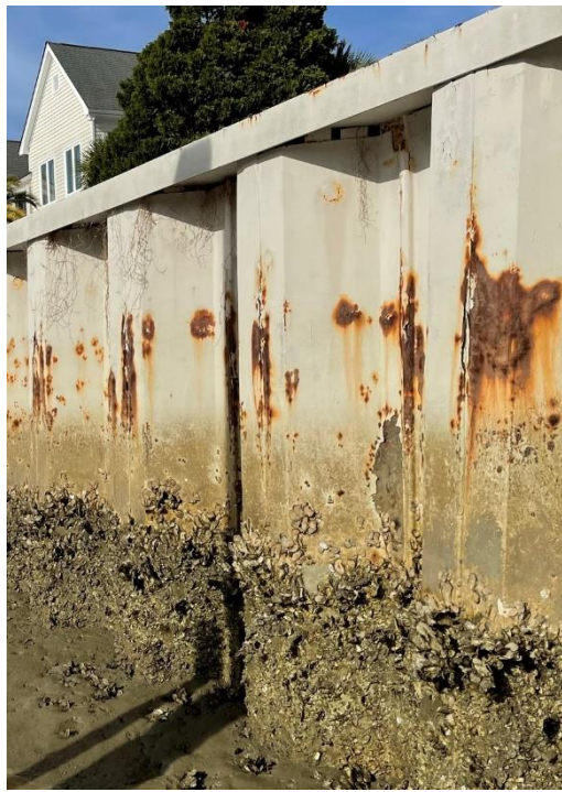
019-closeup view of corrosion and some pin holes Station 22+00
