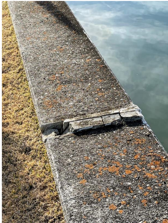
027-cap joint deterioration (typ) Station 44+00
