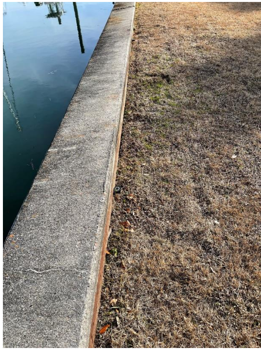
001-backfill subsidence, multiple locations (typ), Stations 59+00/60+00
