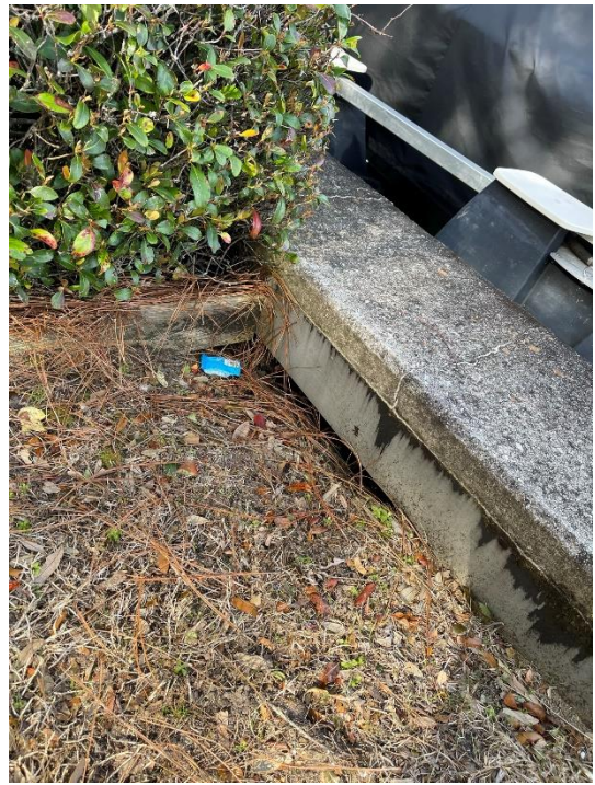
006-backfill subsidence and some soil loss near the back of the wall Station 47+50
