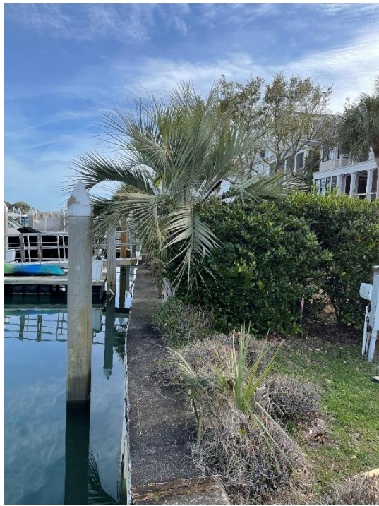
009-heavy vegetation behind the wall Station 36+00
