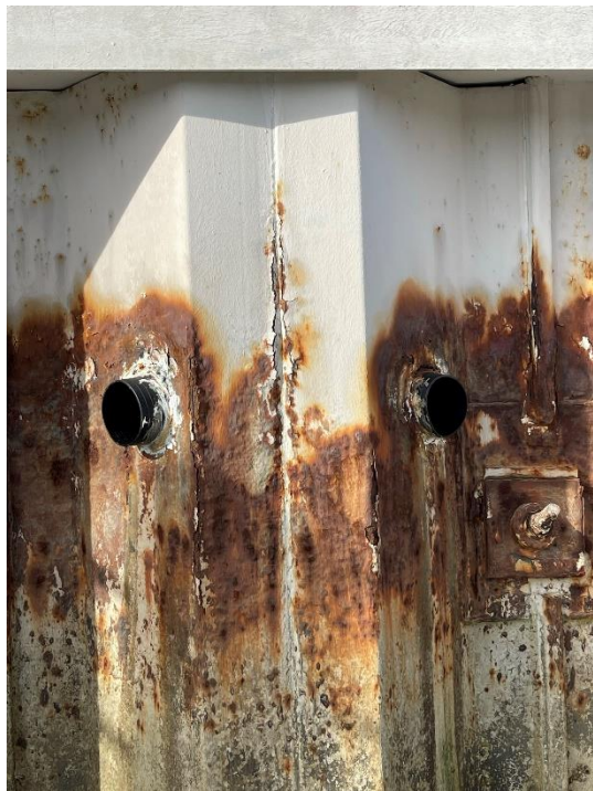
023-closeup, penetrations and corrosion Station 18+00
