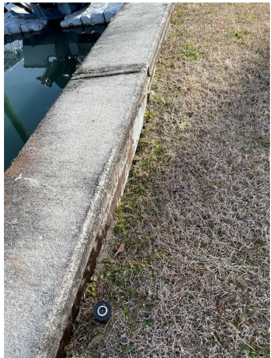
004-backfill subsidence, some soil loss near the wall. Note sprinkle head near the wall Station 57+50
