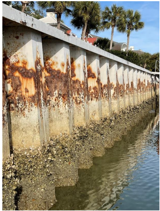
026-corrosion and marine growth, WWI (typical) Station 15+25
