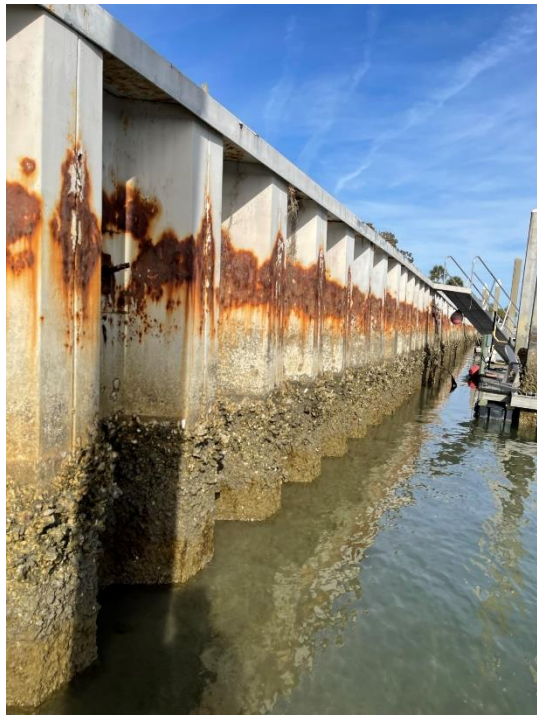
021-marine growth and corrosion, WWI, typical Station 18+00
