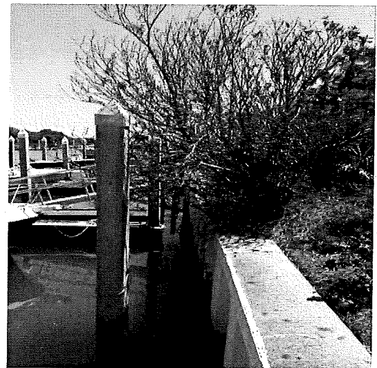
Photo 4. Trees and shrubs have been planted very near to back side of the wall. The wall cap has completely been covered by overgrown shrubs and trees.
