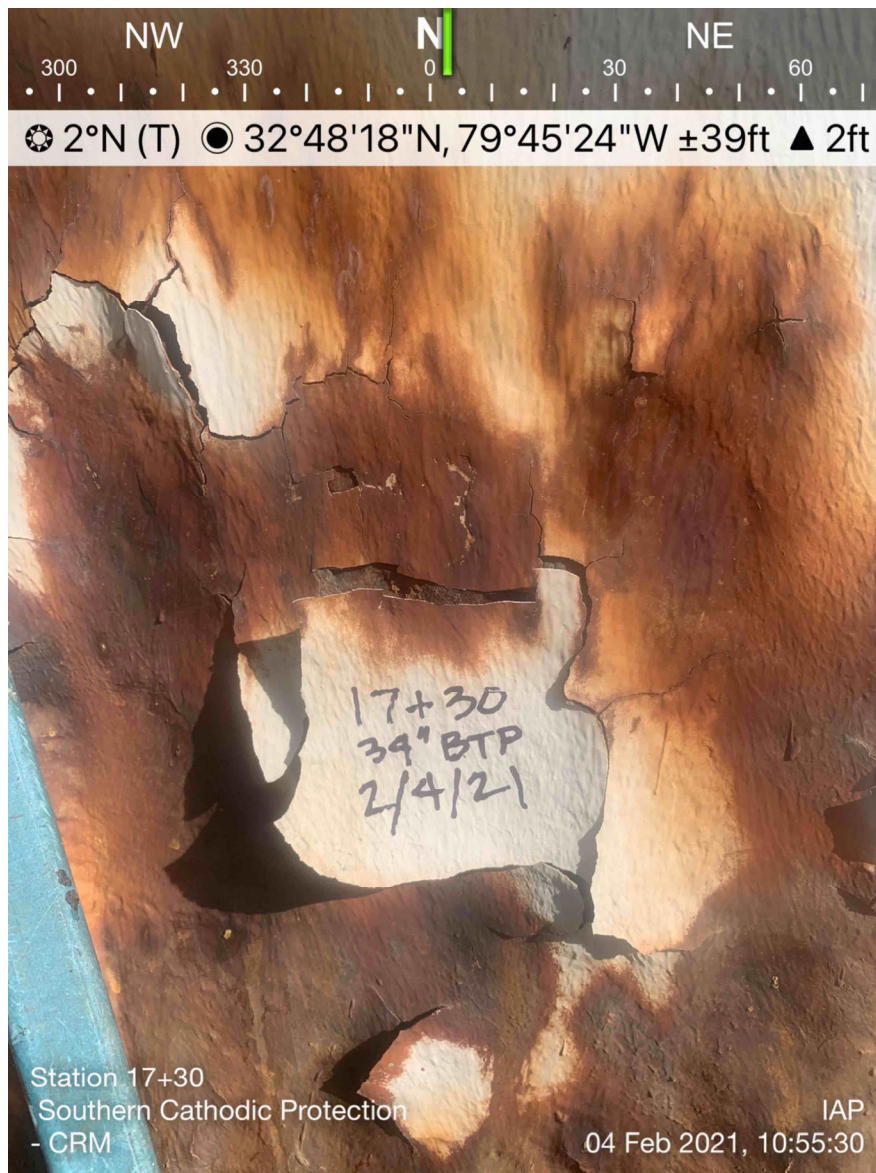
Figure 03: Coating system failure with significant corrosion product scaling in the splash and tidal zones. Location was found on the north wall at Station 17+30.
