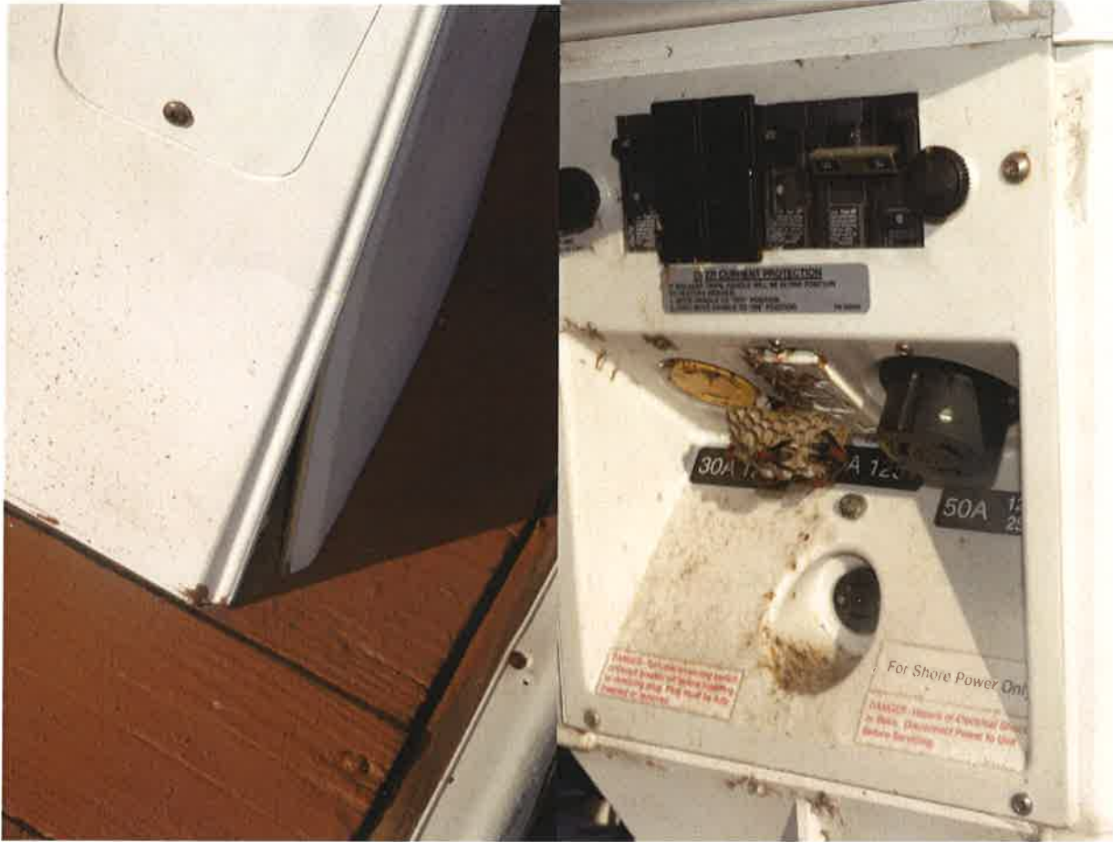
Broken pedestal base and wasps
