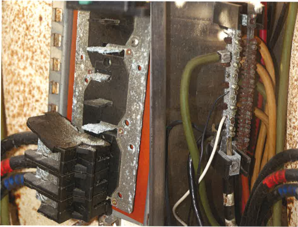
Corrosion at dock A main panel
